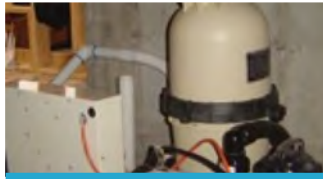
Electric Heater, Pump & Filter
